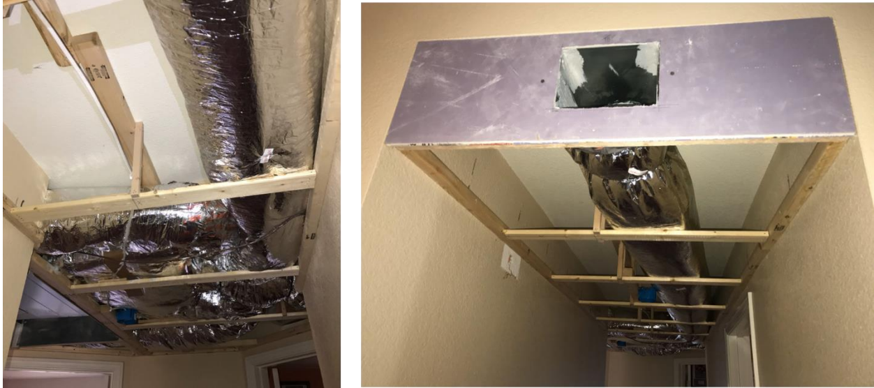
Figure 4. Example install of ducts in conditioned space (Site 1).
